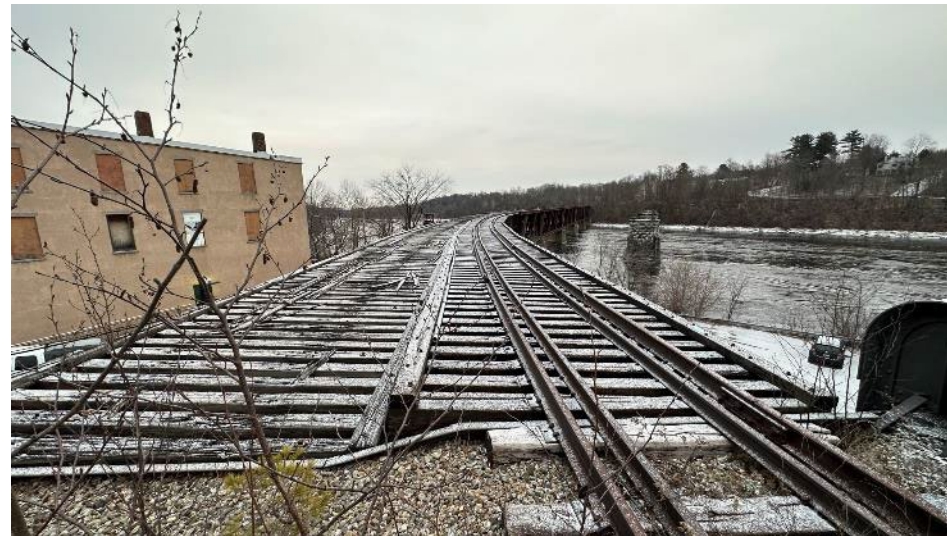
Kennebec River Bridge – Augusta (OOS - 1 Track Removed)
